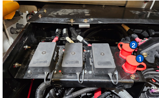
Figure 32 - Remote positive battery posts
