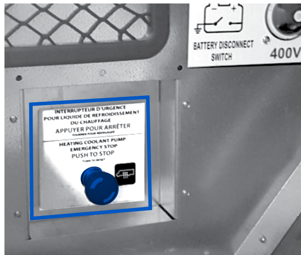
Figure 18 – Heating system emergency stop pushbutton.
