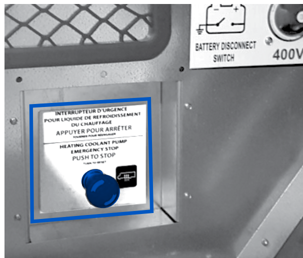
Figure 18 – Heating system emergency stop pushbutton.
