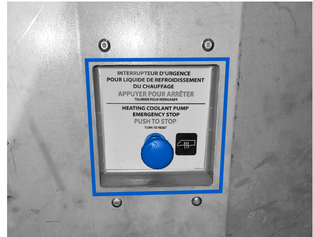
Figure 23 - Heating system emergency stop pushbutton.
